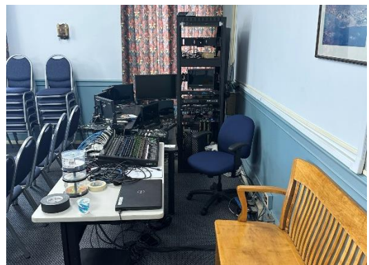
Council Chambers A/V Equipment
