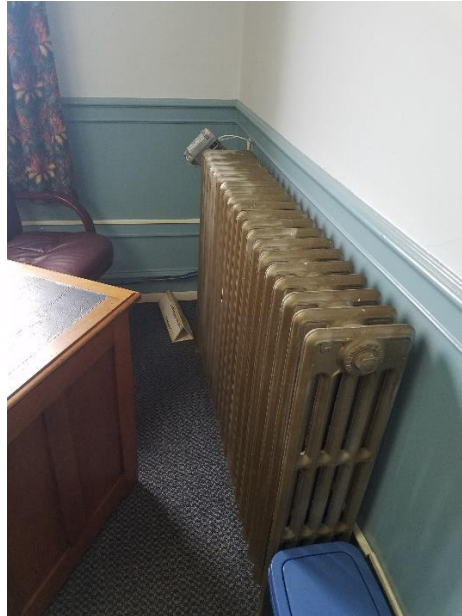
Floor Mounted Steam Radiator
