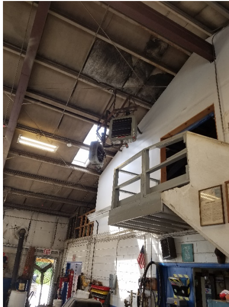
Hot Water Unit Heaters
