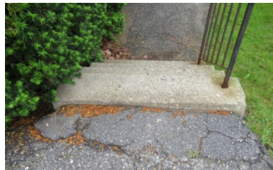
Steps left of entrance (trip hazard)
