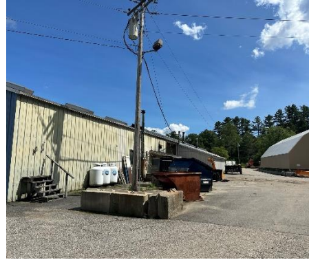
Aerial Utility feed behind DPW building
