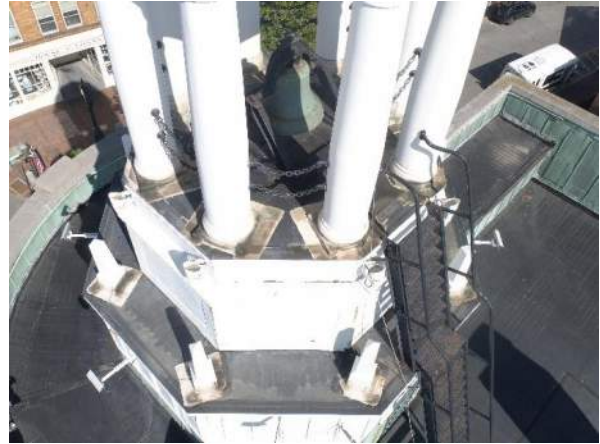
Figure 25: Deteriorated flashing membrane at bell tower penetrations.
