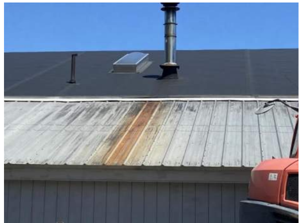
Figure 13: Corrugated metal roof deck with rust staining.
