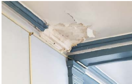
Moisture Damage at Ceiling
