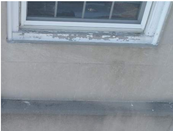
Figure 14: Typical peeling paint at existing wood window frames.
