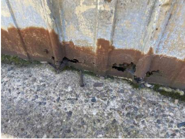
Figure 6: Rust staining and deterioration at the base of the metal wall panels.
