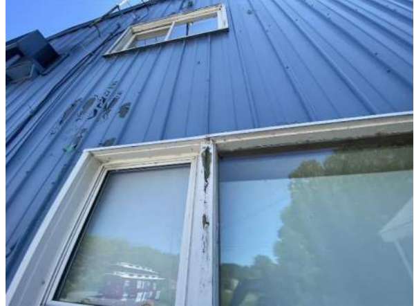
Figure 9: Peeling paint at deteriorated wood framing at window.
