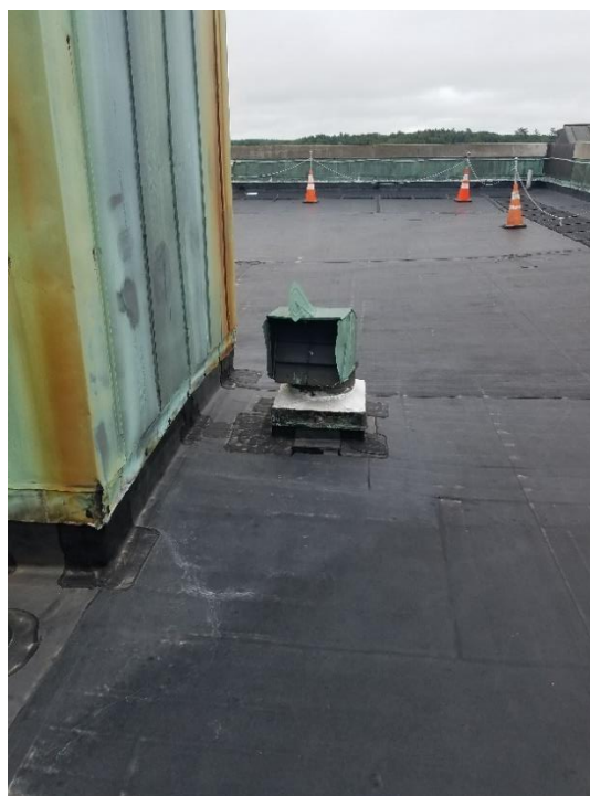
Roof Mounted Exhaust Vent or Fan
