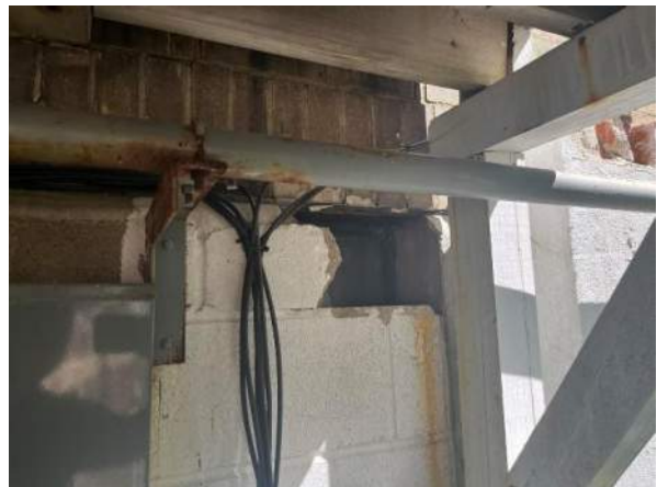
Figure 11: Broken CMU at window infill.
