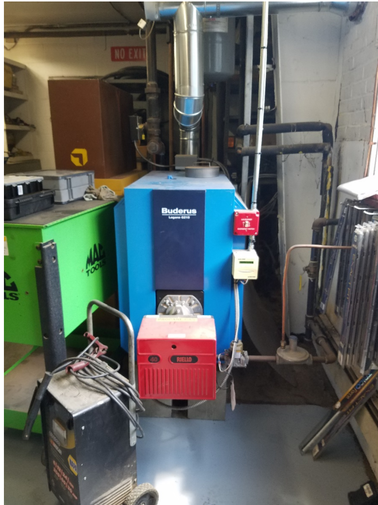
Overall View of Boiler and Burner
