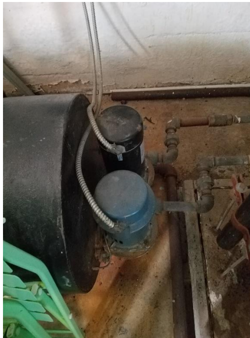
Existing Duplex Condensate Pumps
