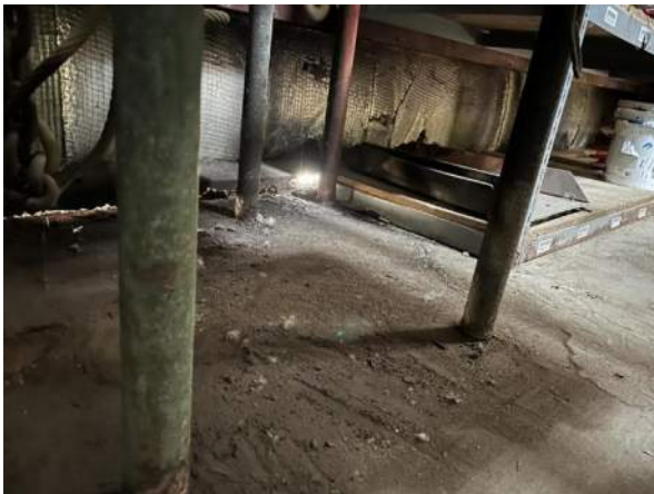
Figure 2: Daylighting at the base of the metal wall panels where water was reported to pool.
