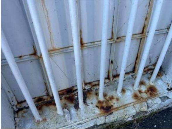
Figure 12: Typical cracked glass and rust deterioration at original steel windows. Note the cracked and spalling concrete.
