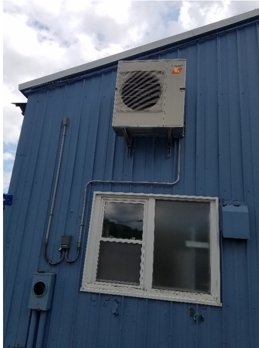
Wall Mounted Outdoor Condenser
