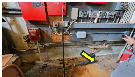
Boiler Room Drainage Piping
