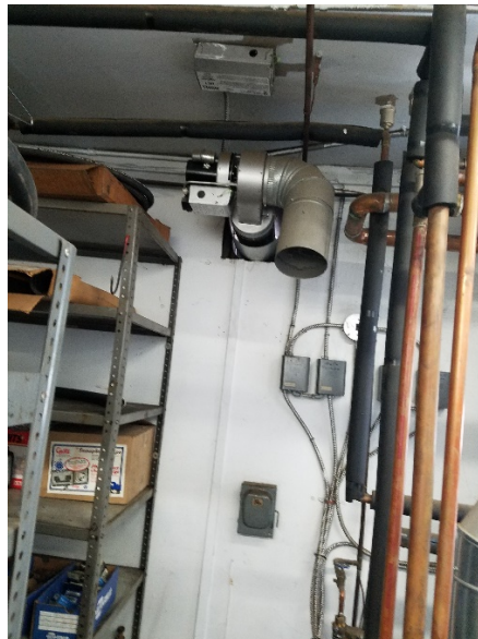
Boiler Room Combustion Air System
