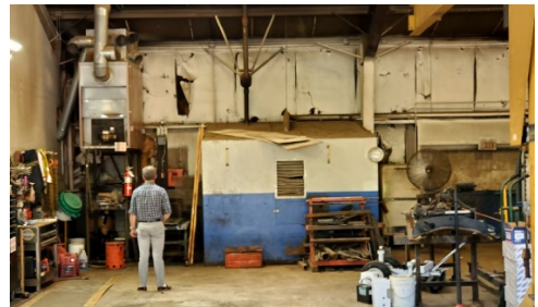
Exposed Insulation in Shop Area
