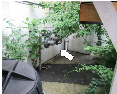
Gas service entrance
