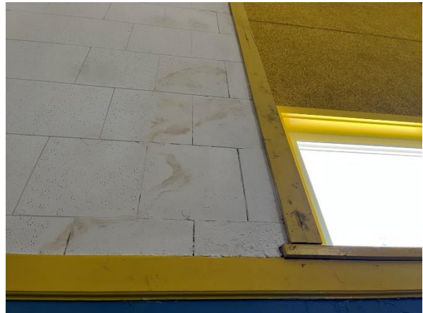
Figure 3: Stained interior finishes at the gymnasium adjacent to window locations.
