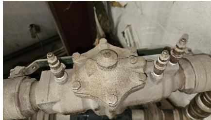
Backflow Preventer for Hose Station
