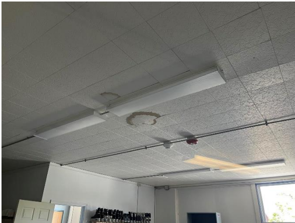
Figure 2: Stained ceiling tiles at the top floor.
