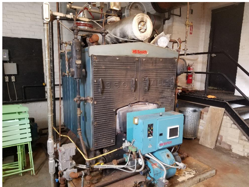
Overall View of Boiler and Burner
