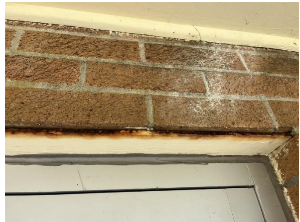
Figure 7: Rusted steel lintel above door location.
