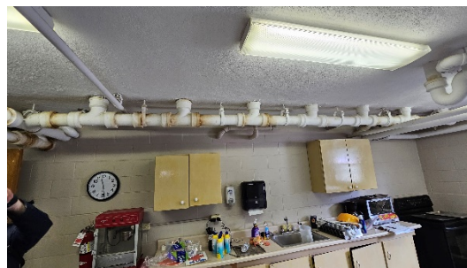
Typical Cast Iron Piping in Break Room
