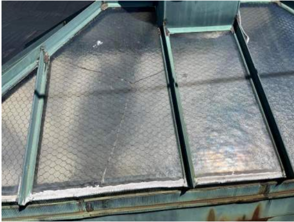
Figure 20: Cracked glass at the copper and wire glass skylight.
