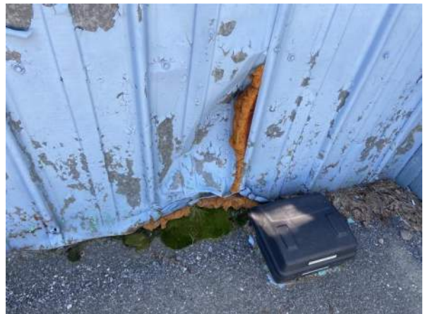
Figure 5: Dented metal wall panel and exposed insulation, with typical peeling paint.
