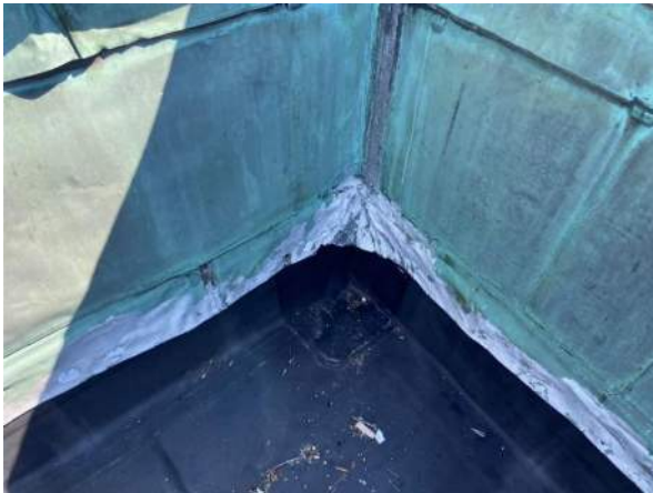
Figure 22: Previous repairs at the copper parapet cladding include aluminum coating.
