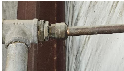
Copper Supply Pipe to Building
