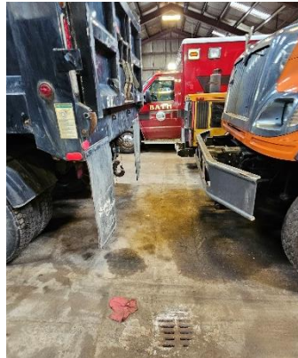
Typical Garage Floor Drain
