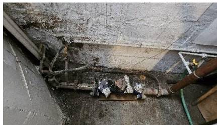
Water Service Meter
