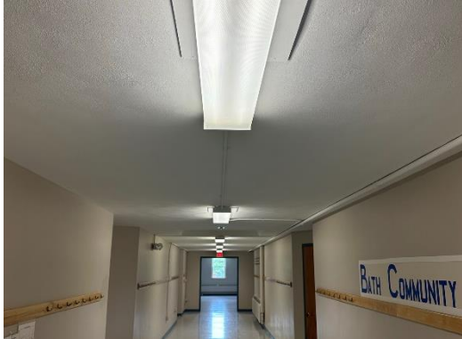
Surface mounted light fixtures
