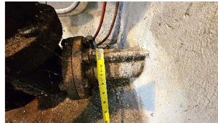
3-inch Water Service Pipe
