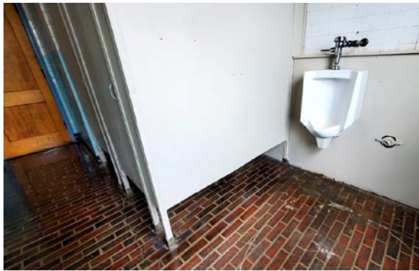
Noncompliant Toilet Room
