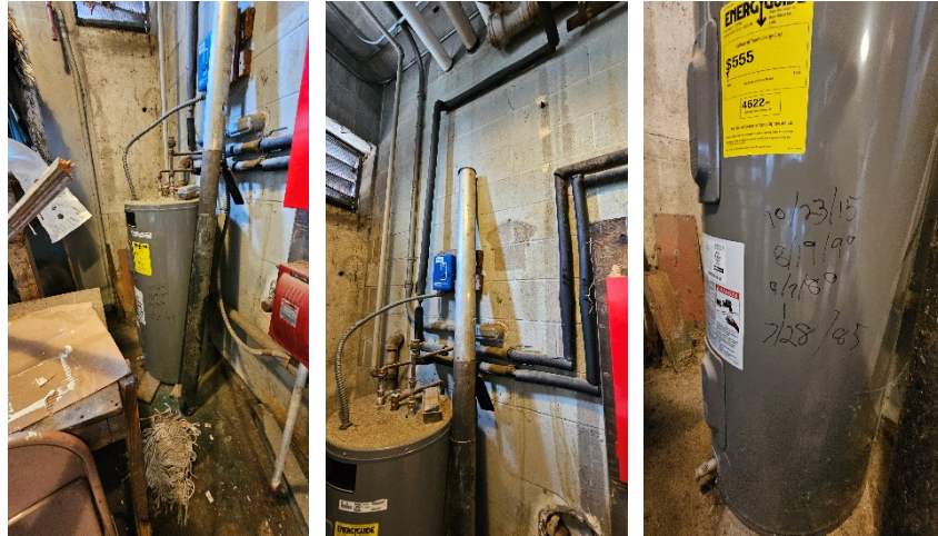
Electric Water Heater
