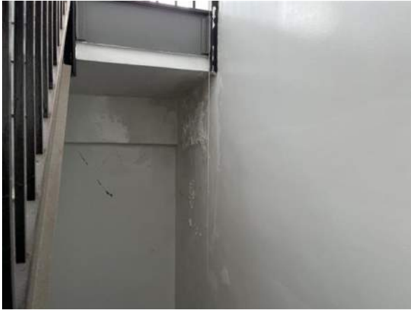
Figure 4: Peeling/bubbling paint at Leak Location #2.
