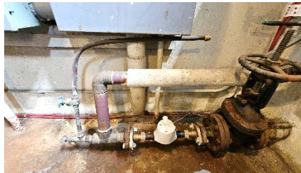
Water Service Entrance
