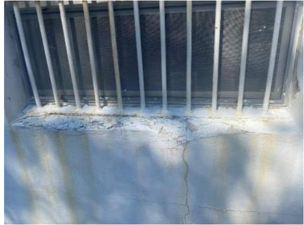
Figure 9: Typical cracked/spalled concrete at basement level windows. Note the steel security bars within the concrete opening.
