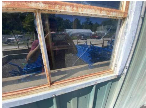
Figure 11: Steel window with cracked glass.
