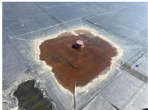
Figure 19: Ponding water at the roof drain.
