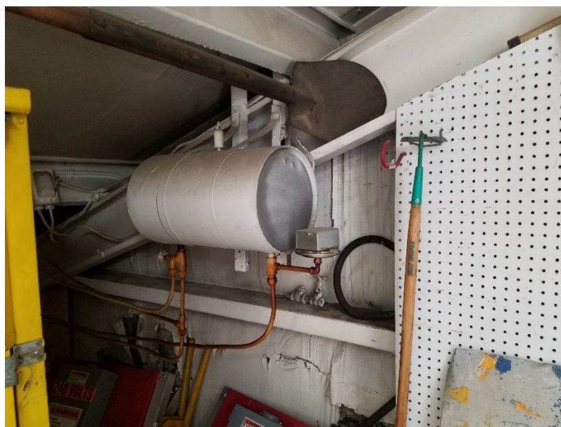
#2 Fuel Oil Day Tank
