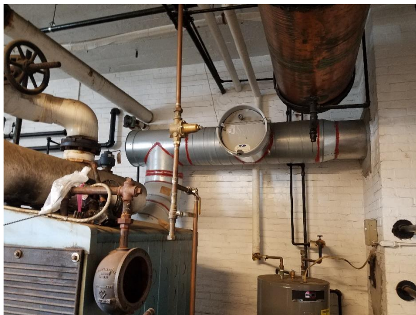
New Boiler Breeching
