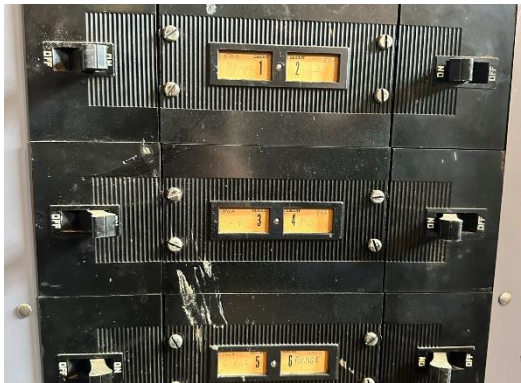
Outdated distribution circuit breakers
