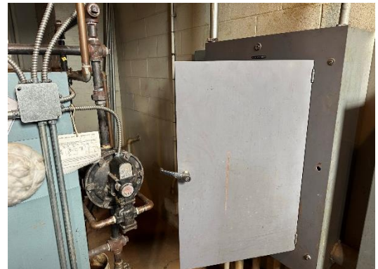
NEC 110.34(A) Clearance Violation
