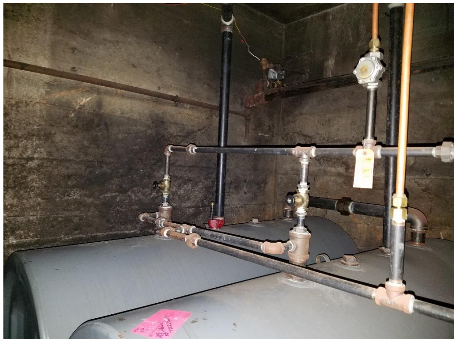
Oil Tank Fill and Vent Piping
