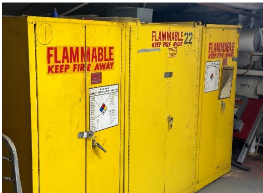
Flammable Cabinets in Mezzanine
