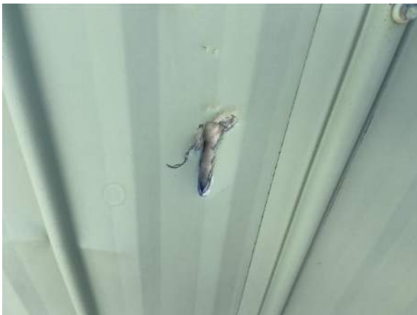
Figure 4: Open/torn sheet metal panel.
