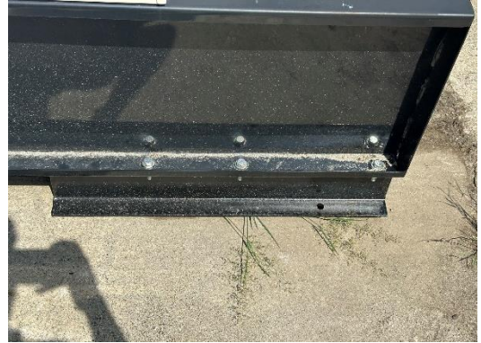
Lack of bolted anchor connections to slab for generator
