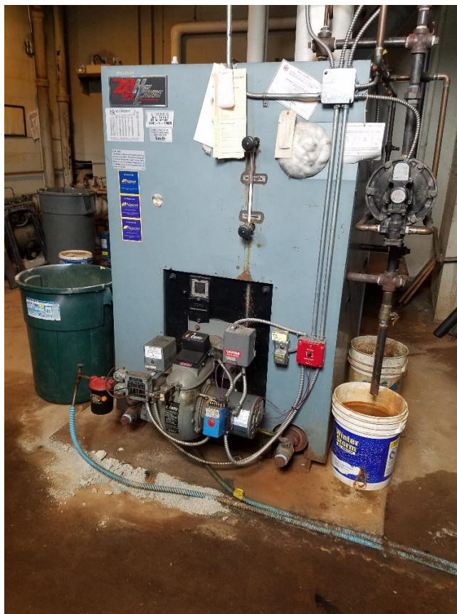
Overall View of Boiler and Burner
