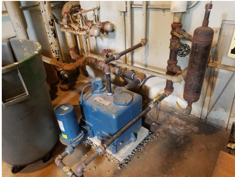
Existing Simplex Condensate Pump
