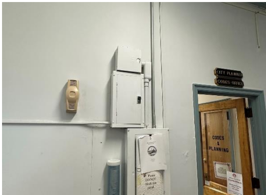
Surface mounted conduit
