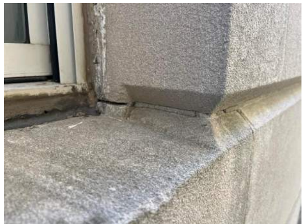
Figure 7: Typical deteriorated mortar joint at limestone.
