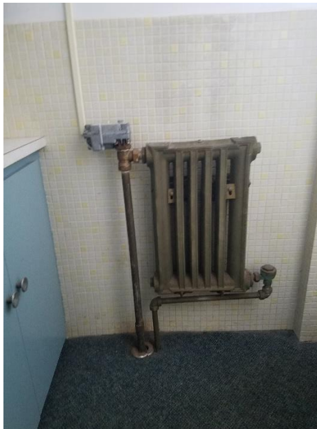
Wall Mounted Steam Radiator
