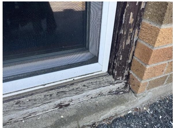
Figure 11: Typical peeling paint at original wood window frames.
