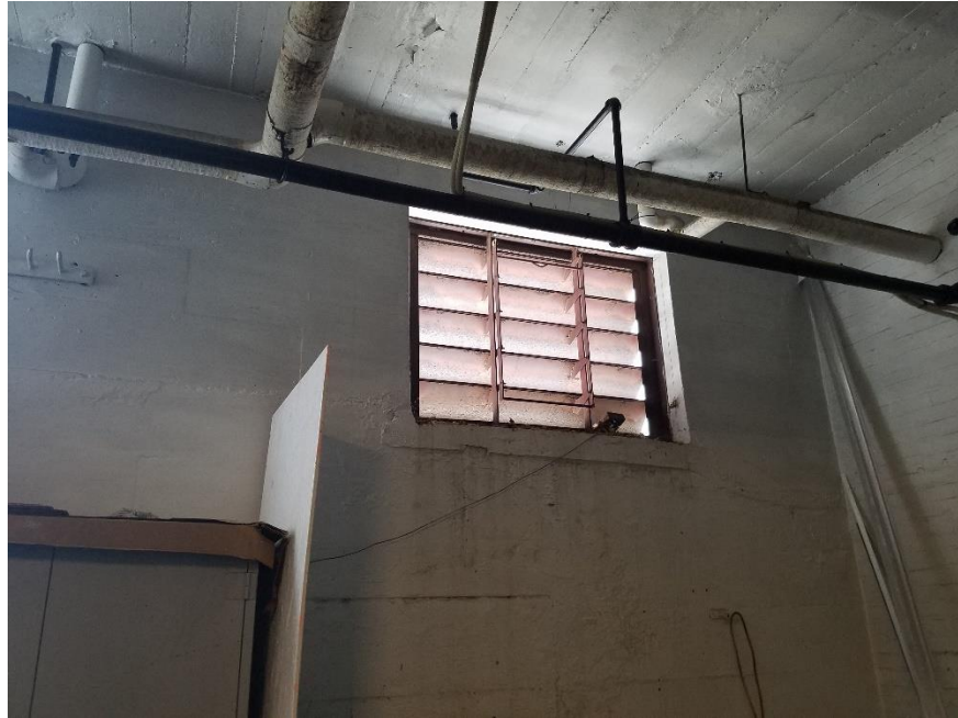
Boiler Room Combustion Air Opening
