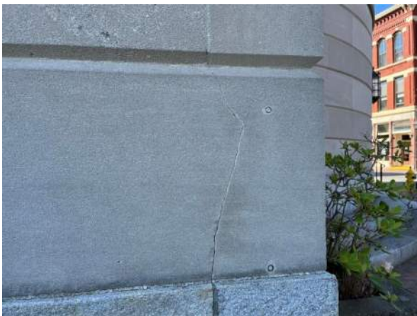
Figure 6: Typical cracked limestone.
