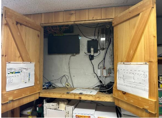
IT equipment in non-approved enclosure
