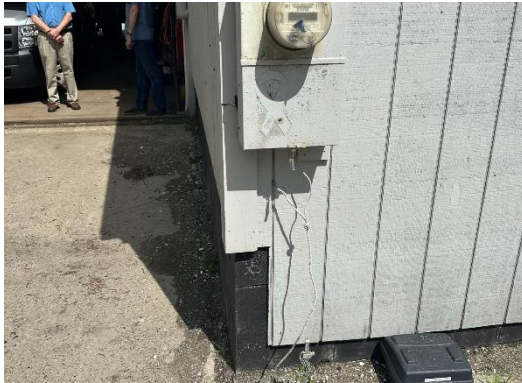
Building mounted utility meter
