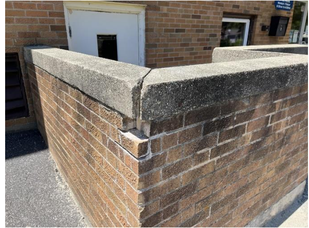
Figure 5: Missing/displaced brick and deteriorated mortar joints at brick masonry retaining wall.
