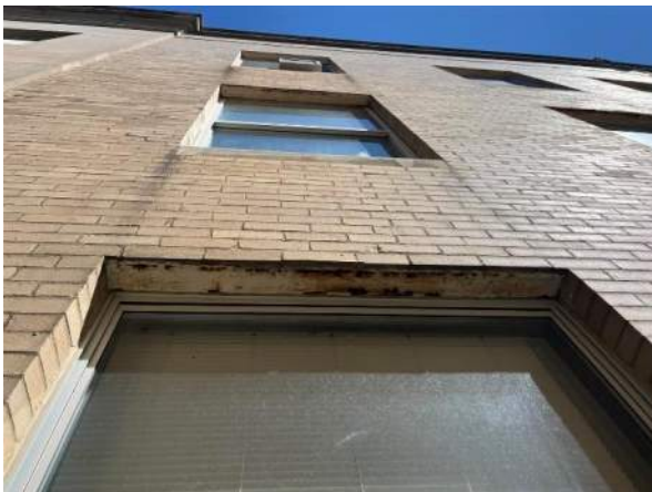
Figure 10: Typical rusted lintel above window location with peeling/blistered paint.
