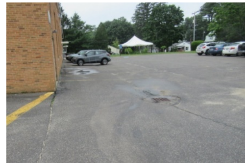
Puddling at east wall of building
