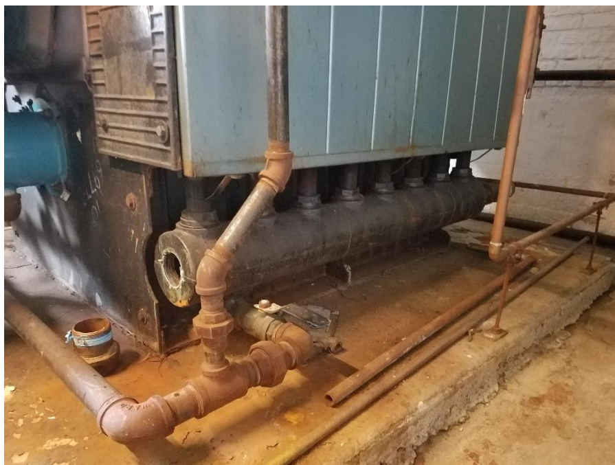
Rust Around Base of Boiler
