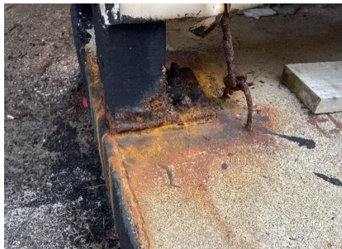
Corroded steel column base.
