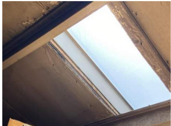
Figure 3: Moisture staining at ceiling adjacent to roof skylight.
