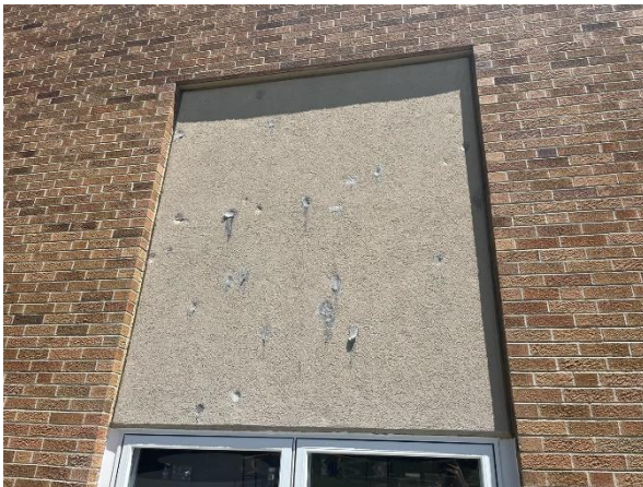
Figure 6: Typical deteriorated EIFS panel.
