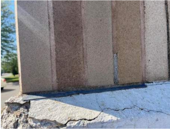
Figure 8: Brick masonry soldier course rebuilt at the corner with copper flashing and weeps. Note the cracked and spalling concrete.
