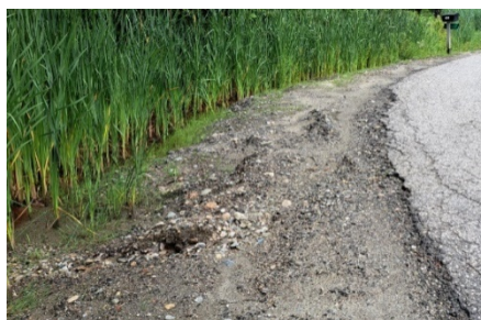
Erosion at pavement edges
