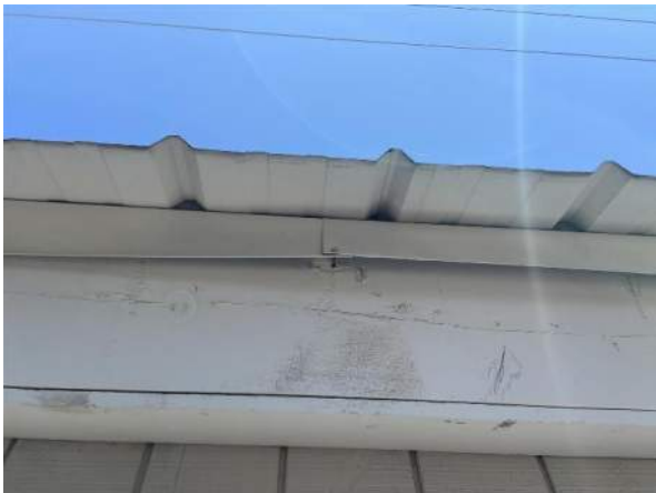
Figure 14: Loose edge metal trim with fasteners backing out.
