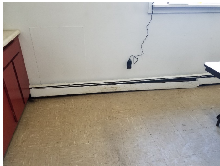
Wall Mounted Hot Water Baseboard Heater
