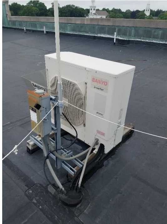
Roof Mounted Condensing Unit
