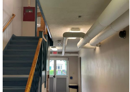
Exit sign obstruction
