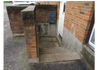
Areaway steps (no handrail)
