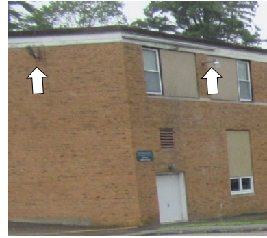
Building mounted site lighting
