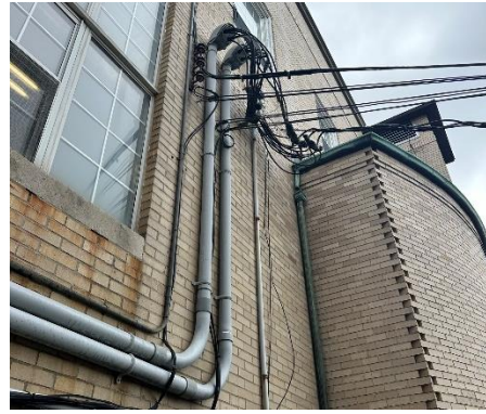
Aerial Utility Feed
