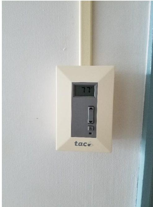
Wall Mounted Temperature Sensor
