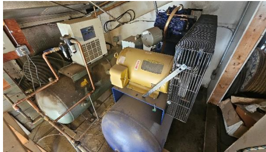
Air Compressor on Mezzanine
