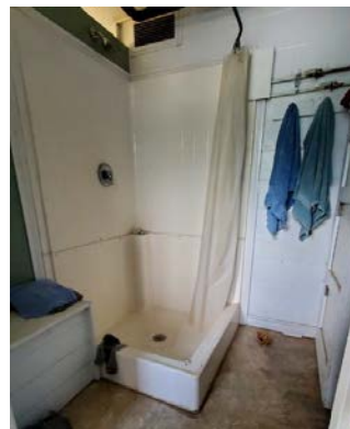
Inaccessible Shower Stall
