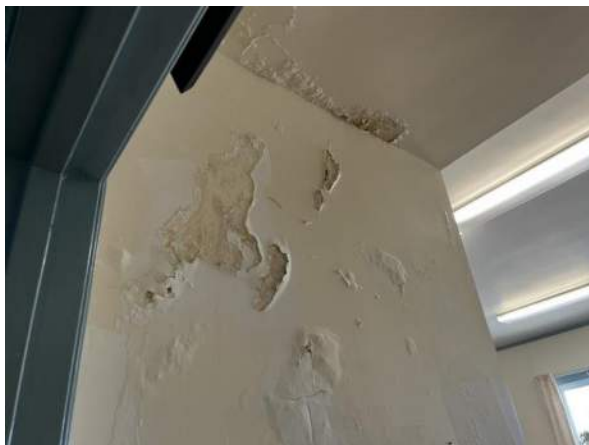
Figure 2: Peeling/bubbling paint at Leak Location #1.
