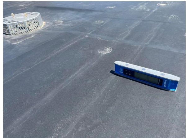
Figure 13: The roof did not appear to be constructed with a slope towards drain locations.
