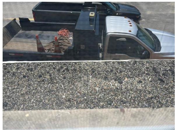
Figure 15: Gravel surfaced roof area.
