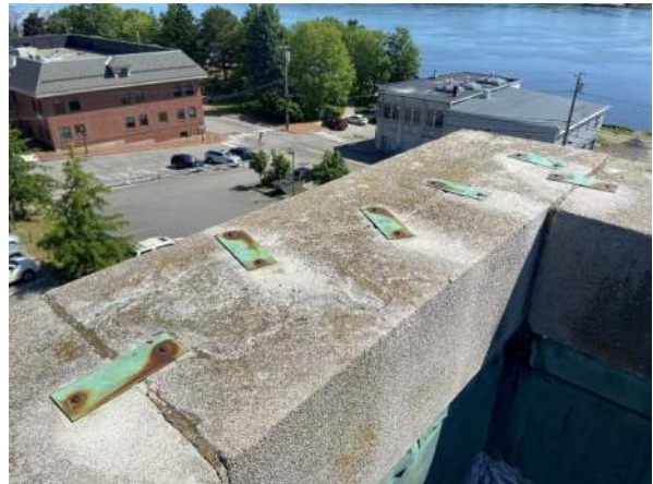
Figure 23: Copper straps at cracked parapet cap.
