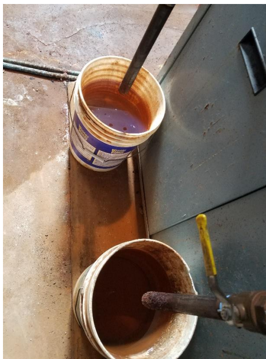
Rust from Boiler Blow Down
