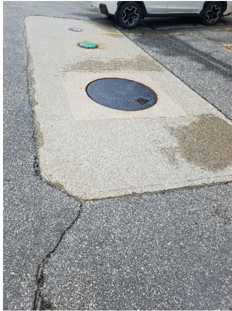
Underground #2 Fuel Oil Storage Tank
