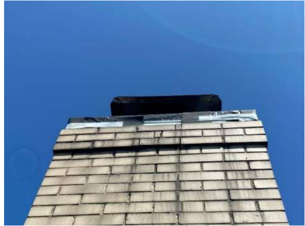
Figure 21: Previous repairs at the chimney cap include a self-adhered membrane and duct tape.
