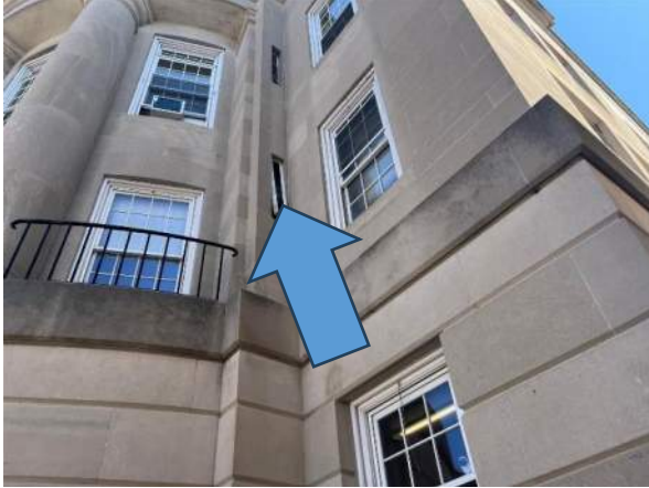
Figure 16: Displaced storm window at the north west elevation.
