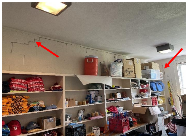
CMU wall Cracks
