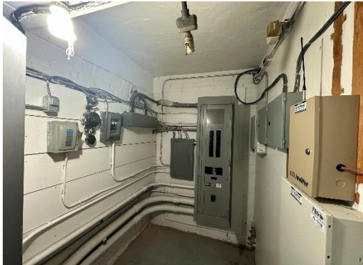
Main electrical room equipment
