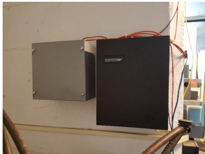
DDC Control Panel
