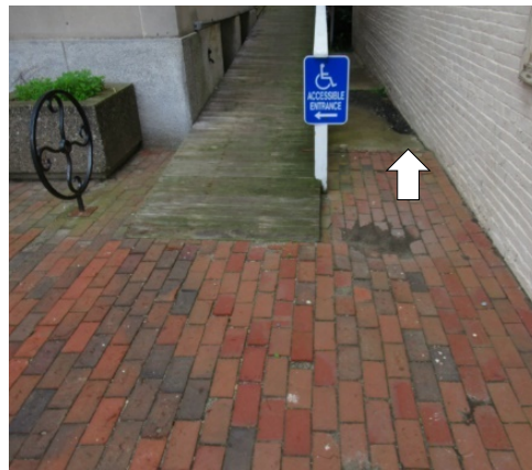
Puddling near ramp
