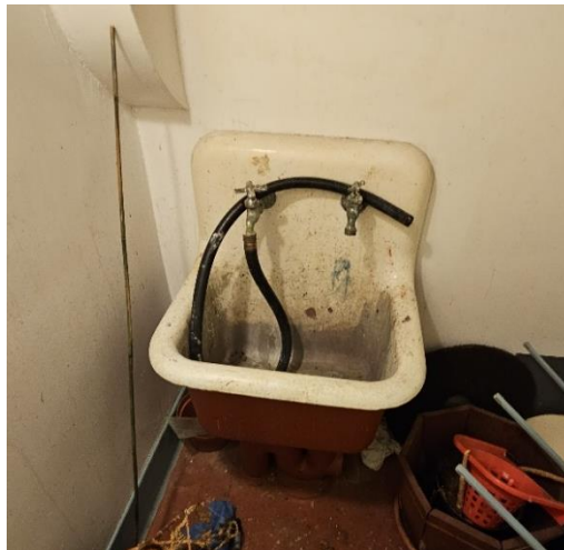
Custodial Service Sink
