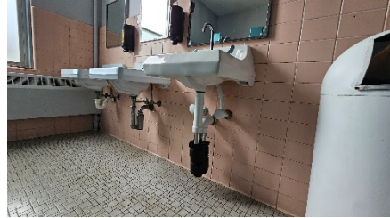
Non-Compliant Trap below ADA Lav
