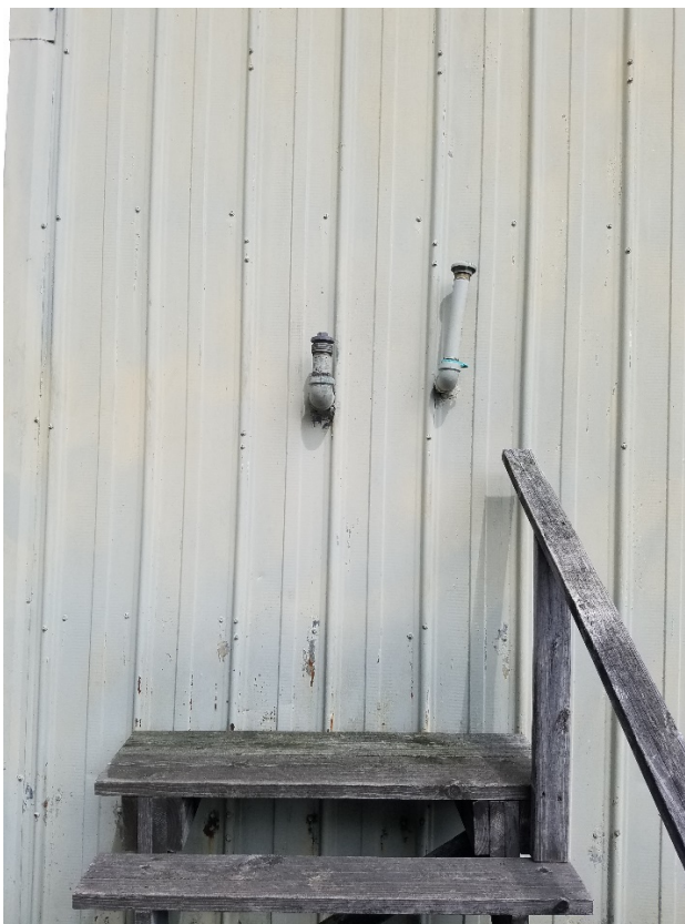
Oil Tank Fill and Vent Lines
