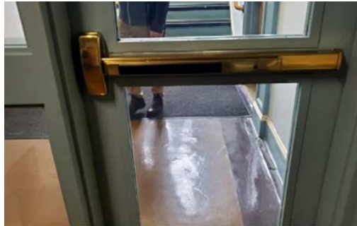
Panic Hardware at Stairwell
