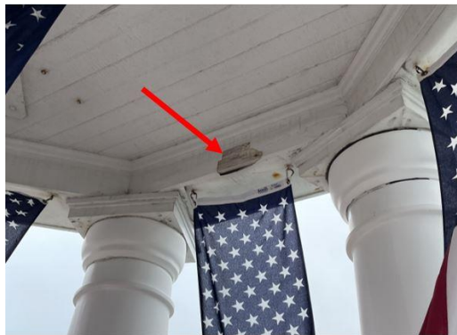
Wood rot at the bell tower
