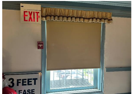
Non-code compliant egress
