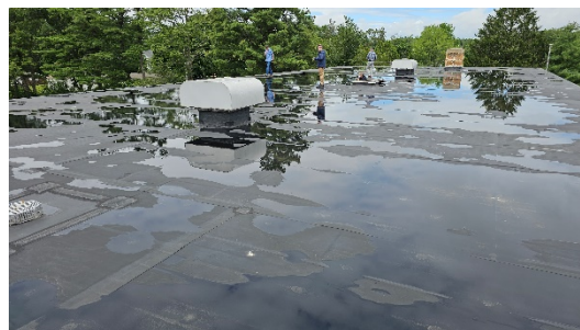
Roof Drain (at left) with Roof Ponding
