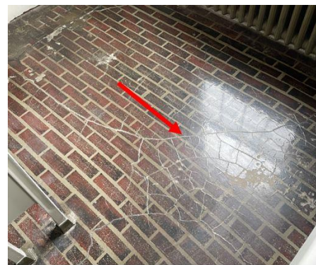
Concrete floor cracks
