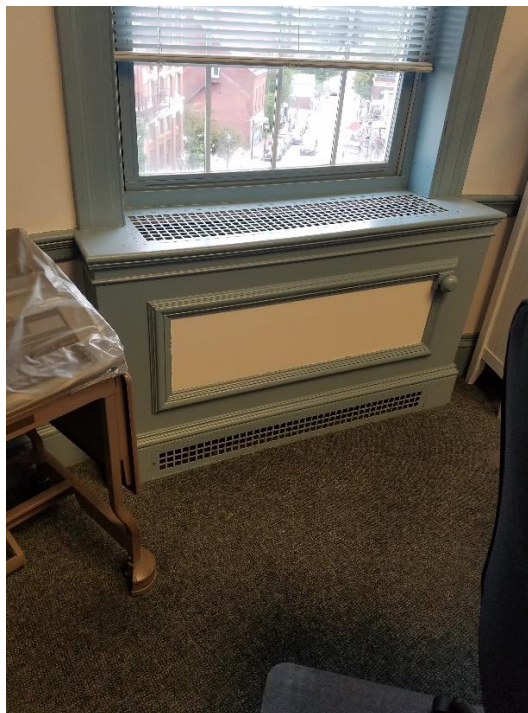
Enclosed Steam Radiator
