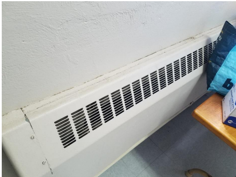
Wall Mounted Steam Baseboard Heater
