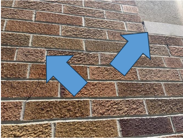
Figure 4: Typical step crack in the brick masonry.
