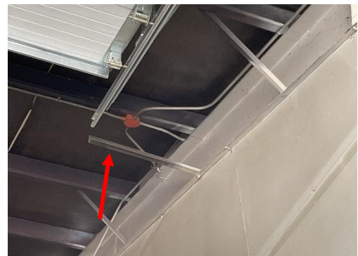
Broken steel kicker angle.
