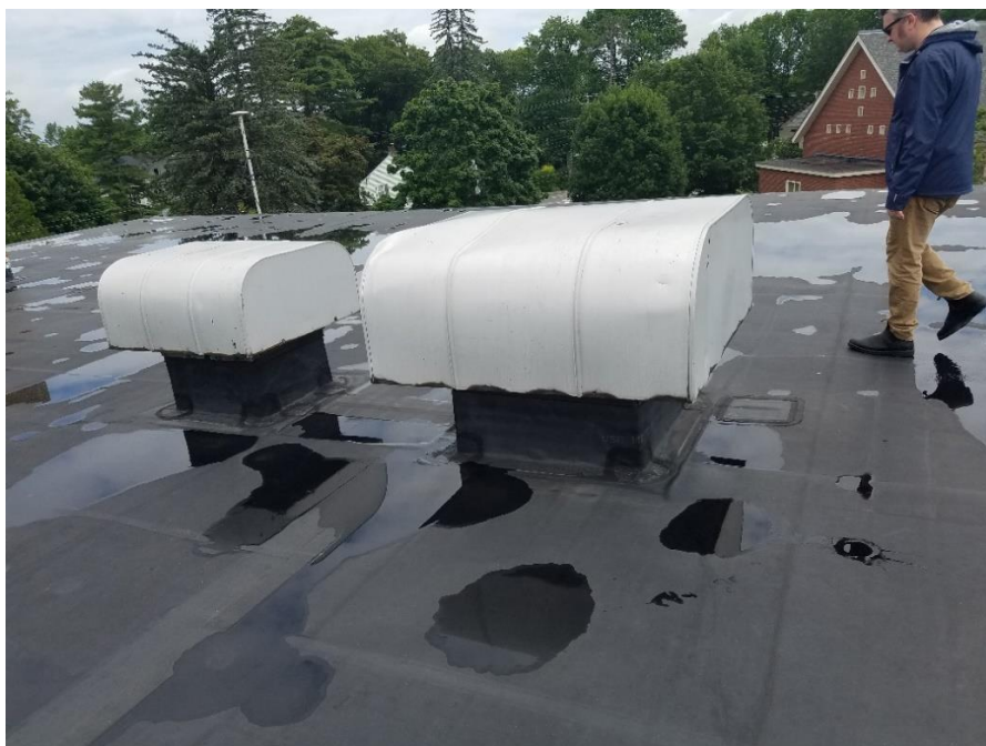
Roof Mounted Exhaust Vent
