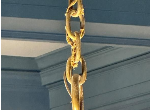
Frayed wiring to decorative chandelier
