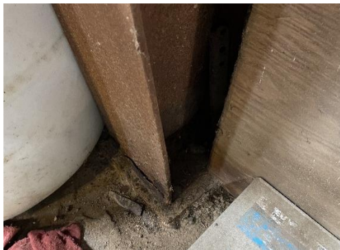
Corroded steel column base.
