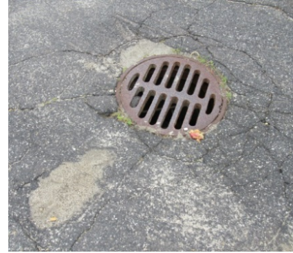
Catch basin rim
