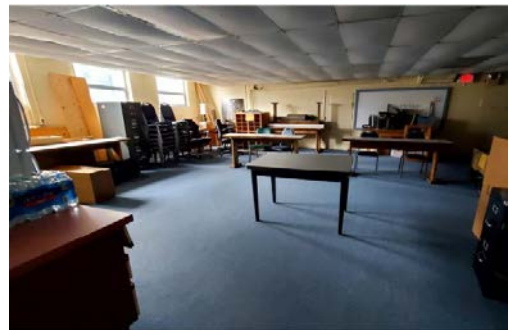
Sagging 2x4 Ceiling Tiles
