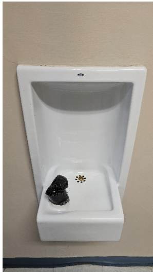
Typical Drinking Fountain
