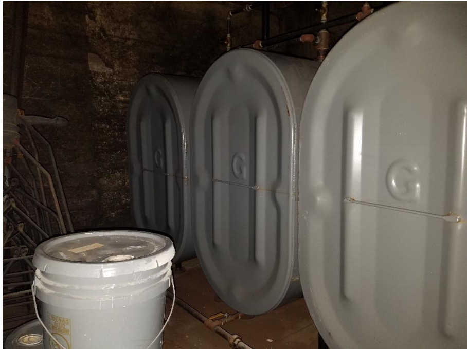
Above Ground Oil Storage Tanks
