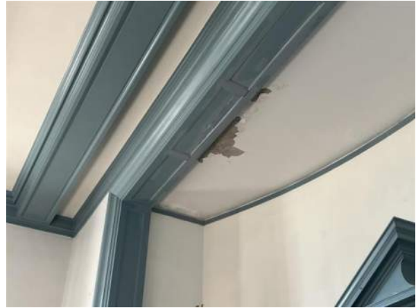
Figure 5: Deteriorated plaster ceiling at Leak Location #3.
