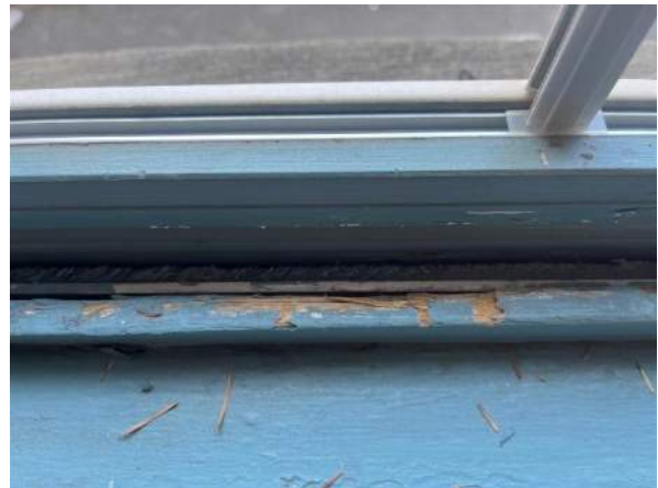
Figure 15: Deteriorated and damaged wood at the interior of the wood composite windows.
