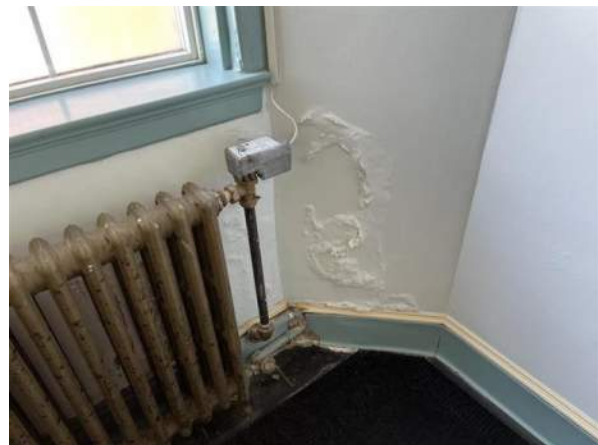
Figure 3: Peeling/bubbling paint at Leak Location #2.
