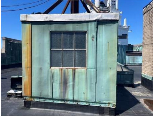
Figure 24: Standing seam copper panel clad penthouse in poor condition.
