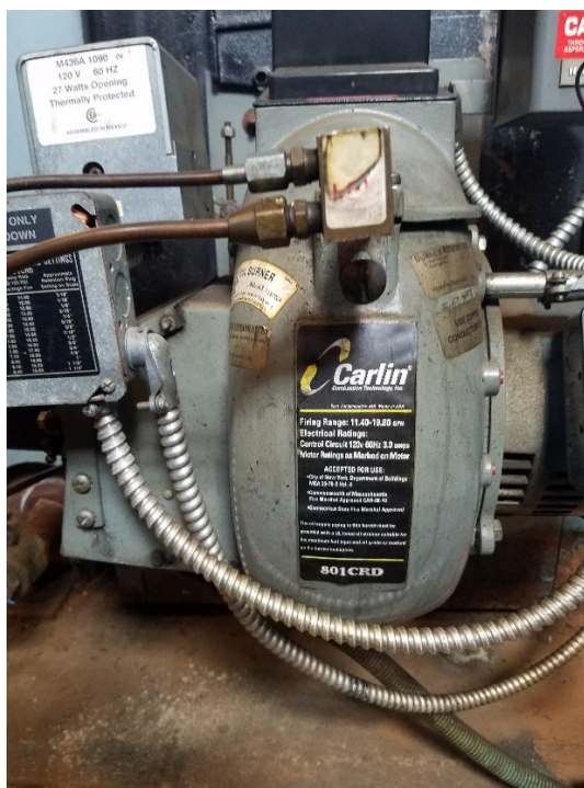
#2 Fuel Oil Burner
