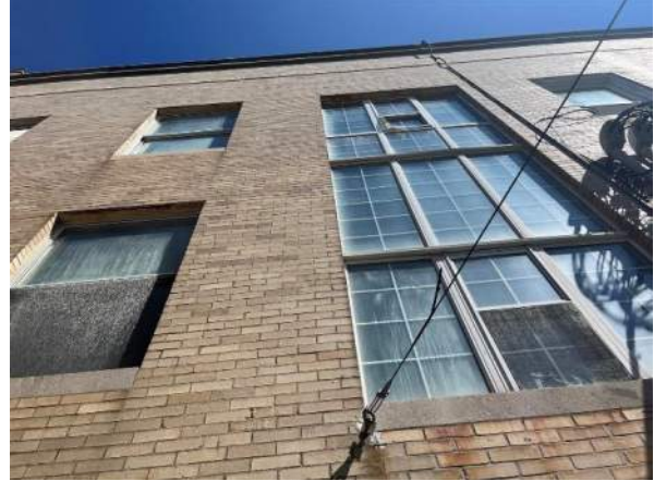
Figure 13: Typical condensation with IGU at the south elevation windows. Note the hazy and foggy appearance of the windows.
