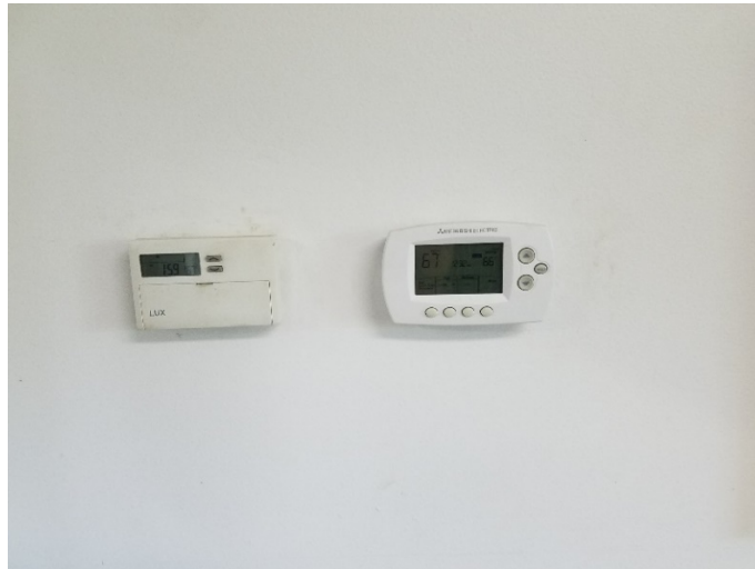
Heating System Thermostat and Heat Pump Thermostat
