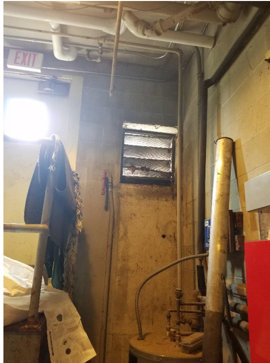
Boiler Room Combustion Air Opening
