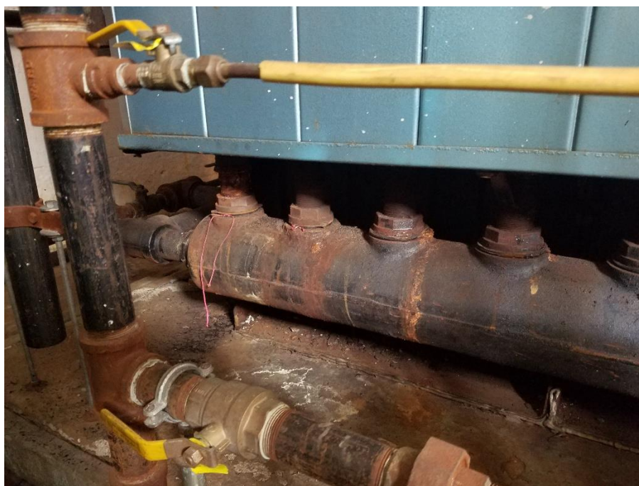
Leaking on Water Side of Boiler
