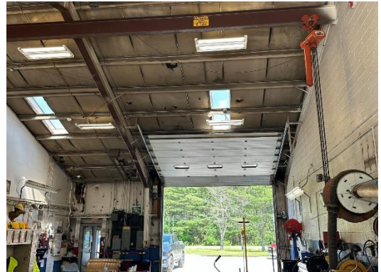
High bay fluorescent light fixtures
