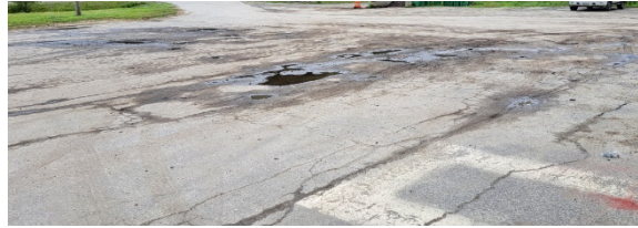
Puddling in paved area – poor pavement conditions
