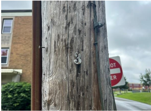
Utility Pole #3 on Sheridan Road
